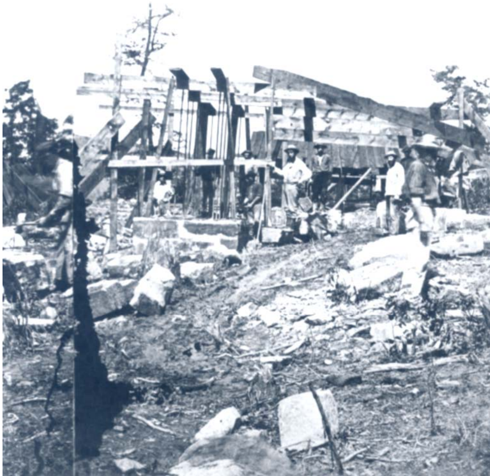
Figure 8. Woodward photograph of the excavation of the Great Petroleum Shaft in 1865. Workmen are busy constructing the framework for the machinery, winches, and pulleys. Photo courtesy of Drake Well Museum (DW 297).
