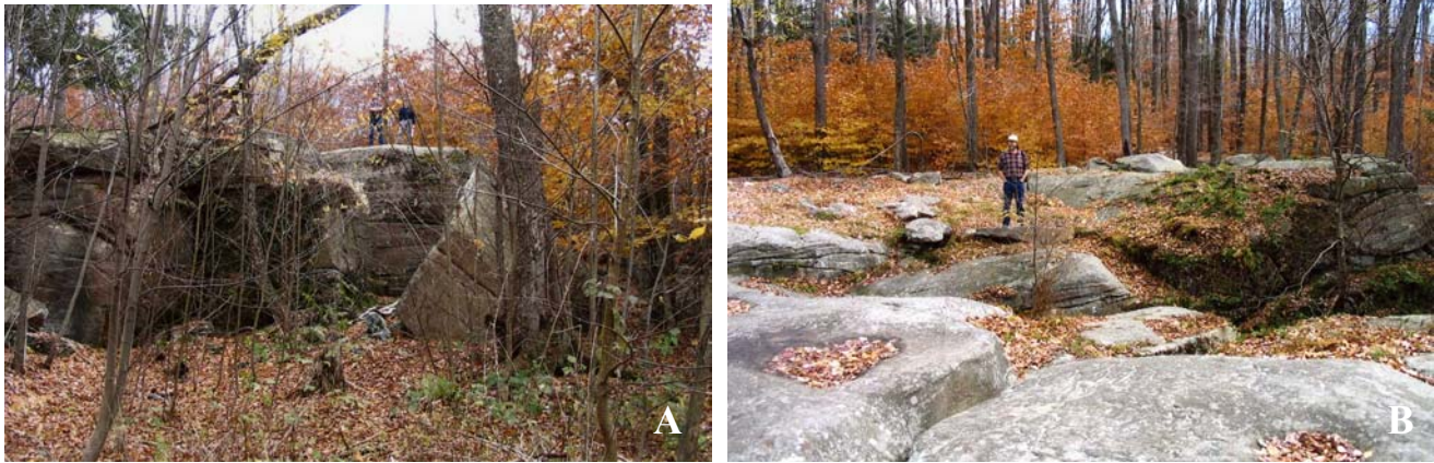
Figure 66. A. The “Rock Garden”; B. Pavement of the “Rock Garden” disrupted along joints.
