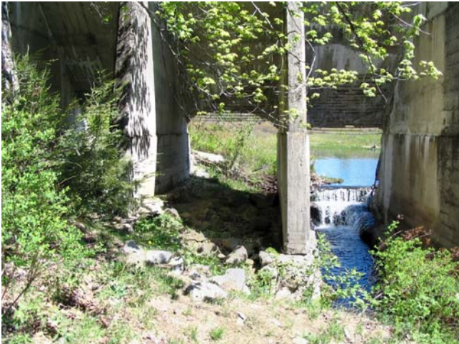
Figure 1-41. Holes blown in Lake Leigh Dam in 1957.
