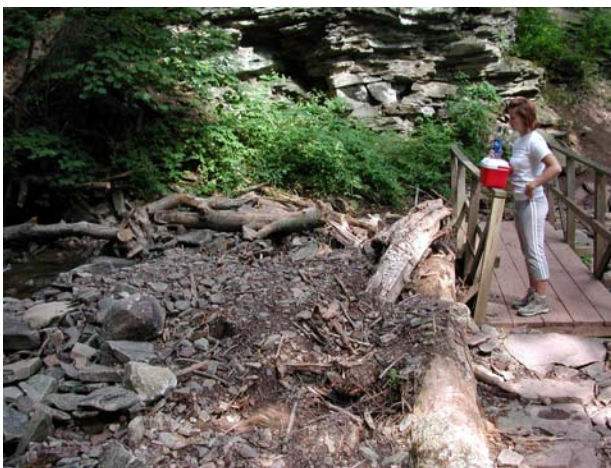
Figure 1-13. Debris and erosion from late June 2006 flood.
